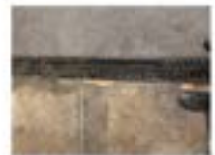
EXISTING FLOOR GRILLES
